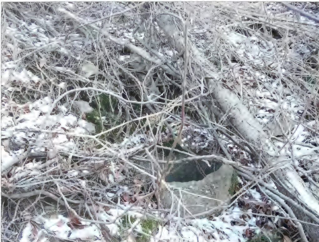
Figure 3.51. Concrete pipe, Battery Kingman. A concrete pipe protrudes through the engineered earthwork northwest of emplacement #2 (Olmsted Center, January 2009).
